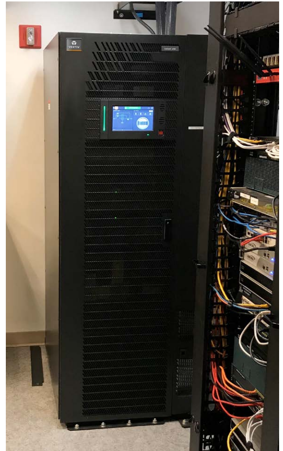
Liebert EXM UPS installed at Pacific Seafood
